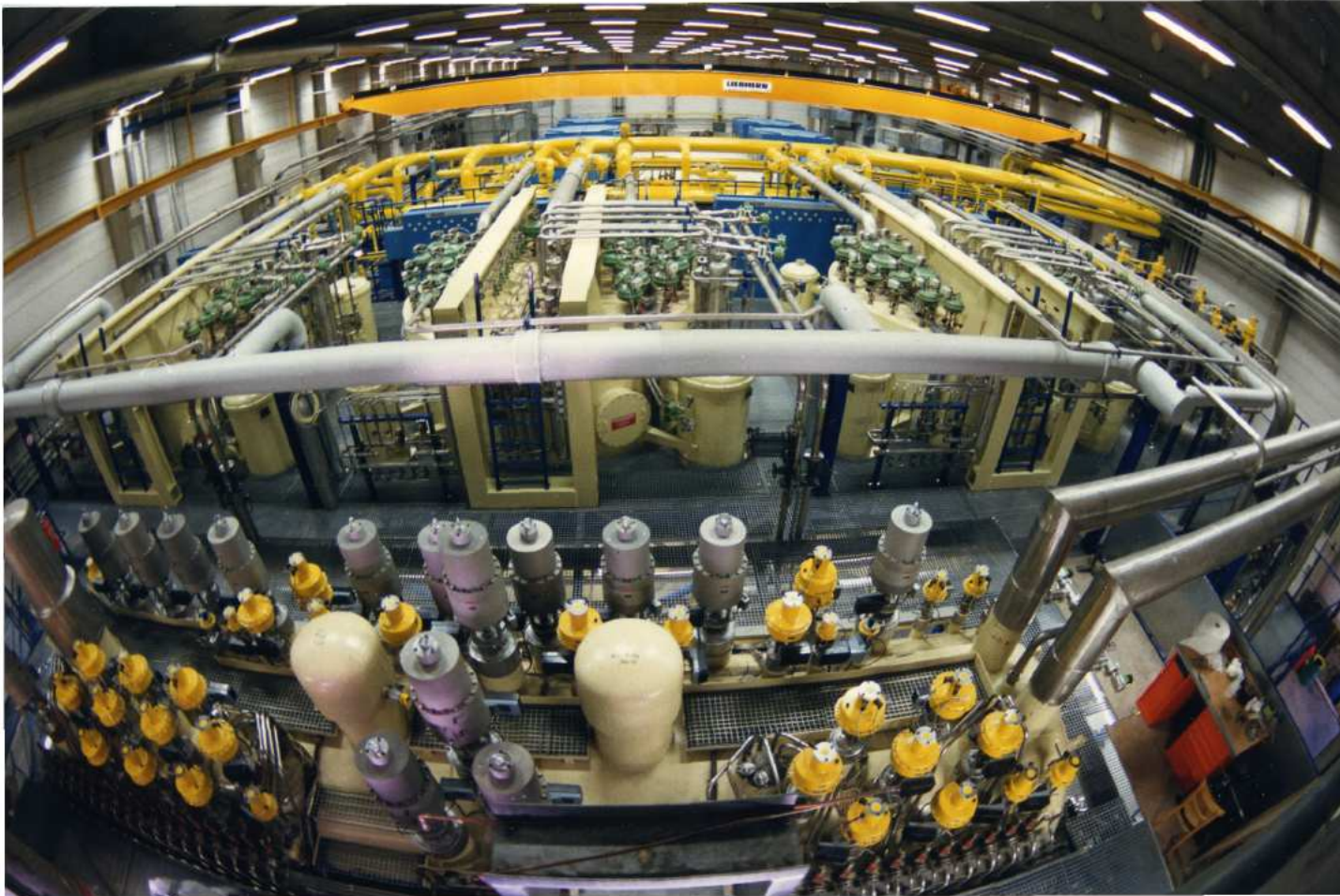
HERA cryogenic plant: 3 cold boxes with 6.3 kW at 4.3 K 20 kW at 40 kW
