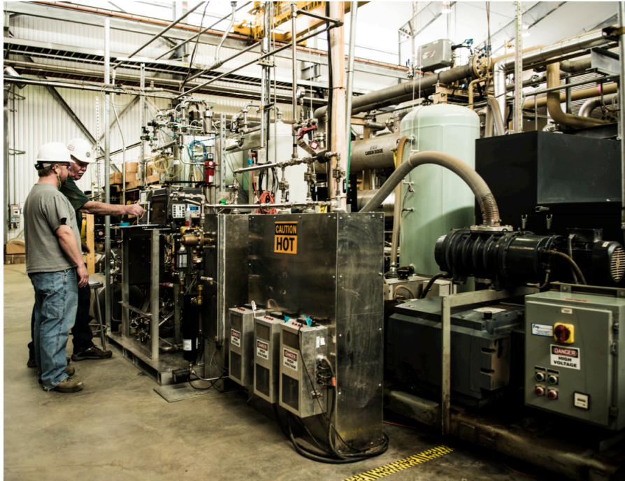
Plant at Colorado
