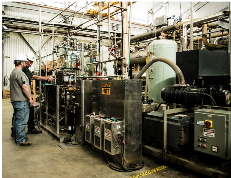
Plant at Colorado
