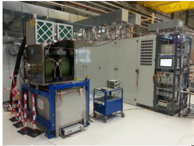
FOS debuncher cavity SAT ongoing.
