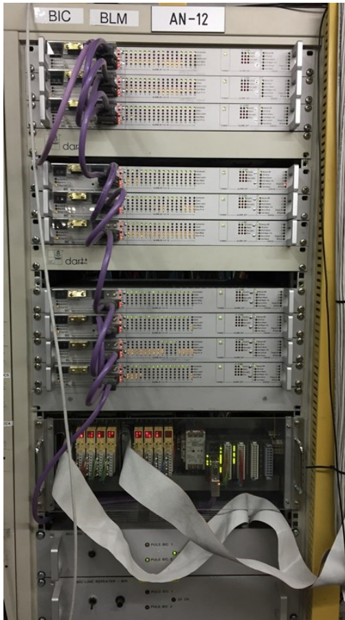
Beam Interlock Concentrator BIC
