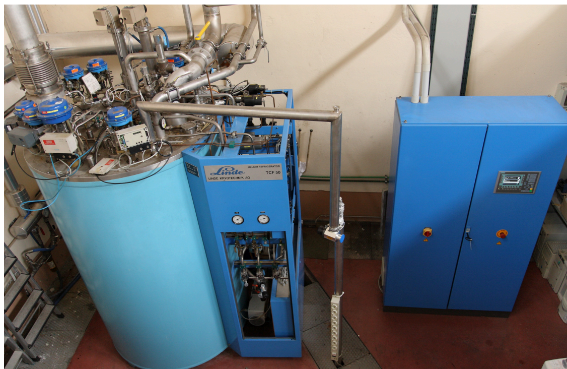
LINDE TCF 50 liquid He liquefaction/refrigeration plant
