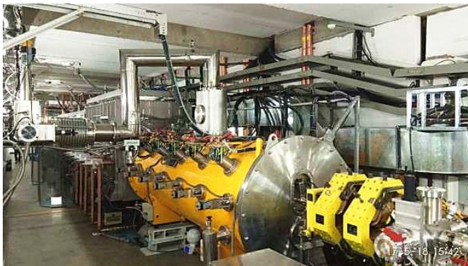
Cryomodule4 @ Main Linac
