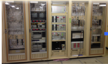
New LLRF Control System
