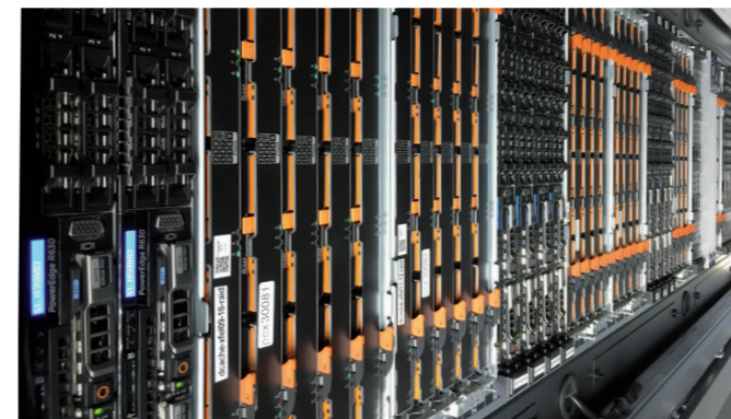
Figure 1 Rack in the computing centre containing IDAF systems
