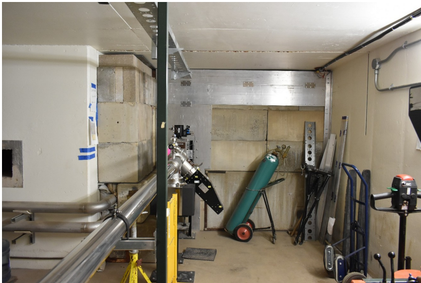
Diagnostic absorber wall
