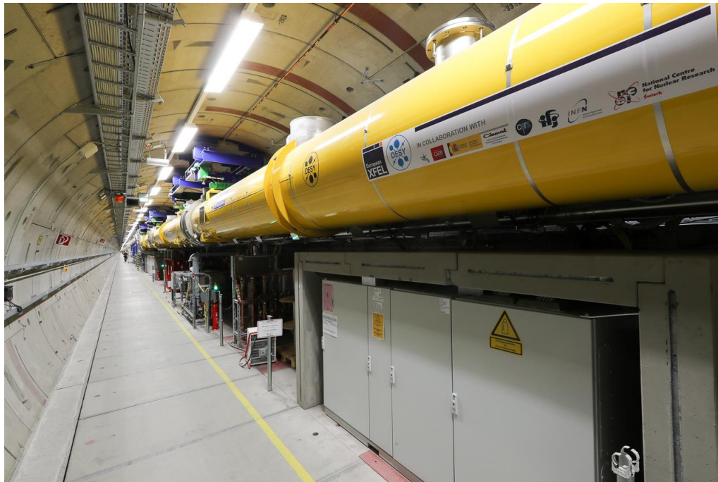
EuXFEL Accelerator Tunnel
