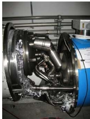
September 19, 2008 Disaster Electrical arc developed in a LHC dipole magnet interconnection
