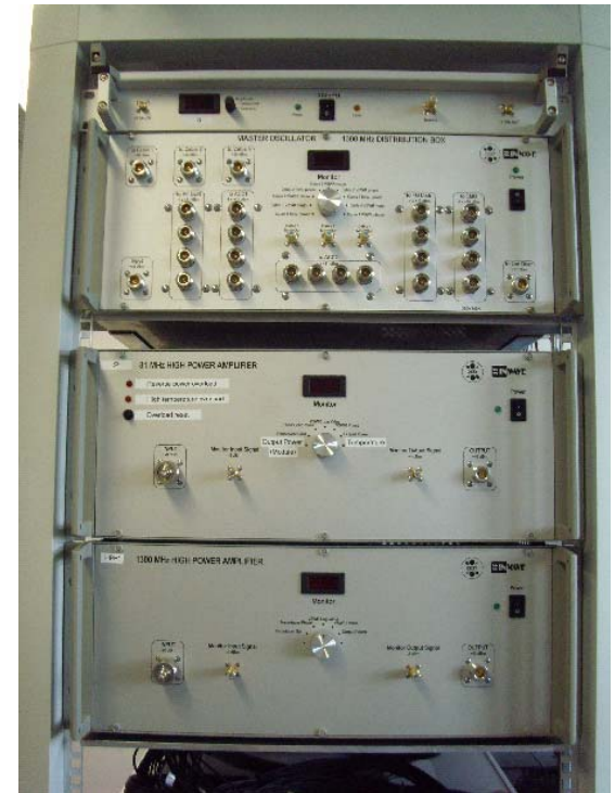
Frequency generation and distribution boxes
