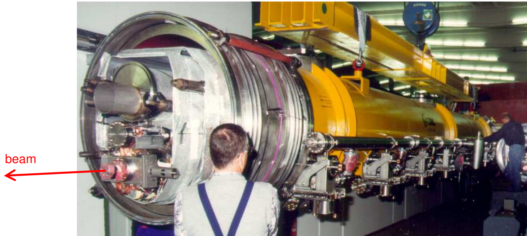
module installation in FLASH (2004)
