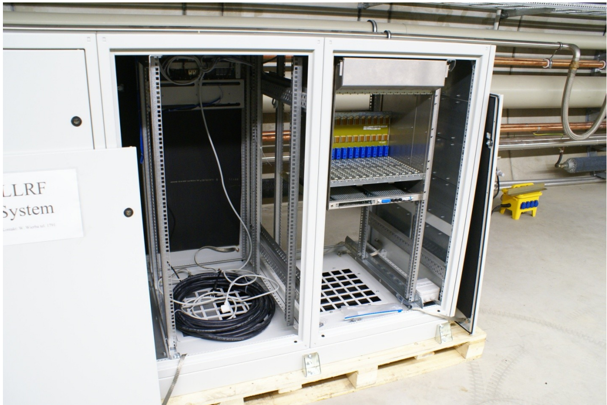
Fig. 17. ‘Container’ with installed ATCA crate.
