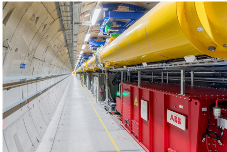
View of the E-XFEL Linac
