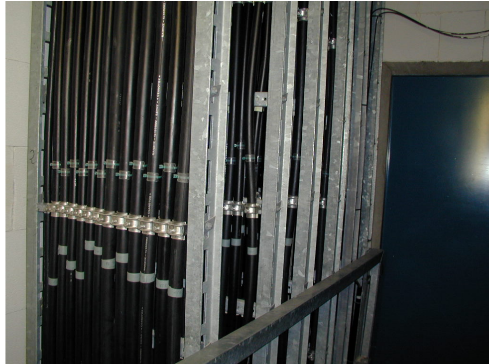
Vertical cable trays in a shaft
