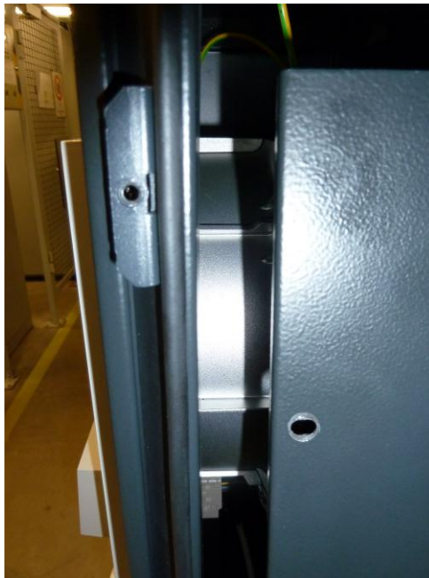
Fig. 1. Rear 'doors' should not be fixed with screws.
