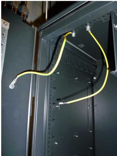
Fig. 10. Such a cables with connectors are not sufficient for EMI grounding.
