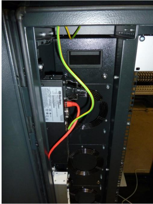
Fig. 7. Cooling Unit has no rubber dampers to prevent vibrations propagation.
