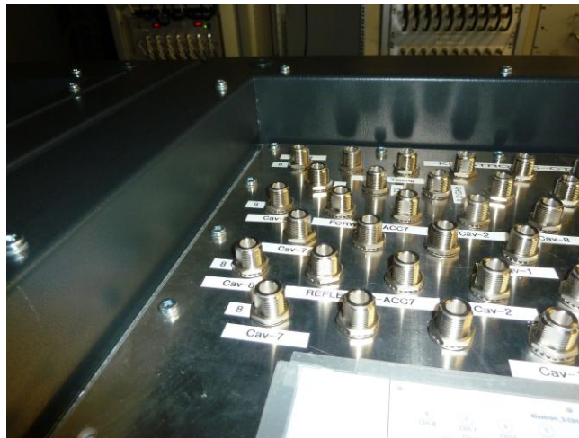
Fig. 6. More screws should be used (~2 times) to fix frame to the top cover. The patch panel is fixed properly, bigger washers are necessary.
