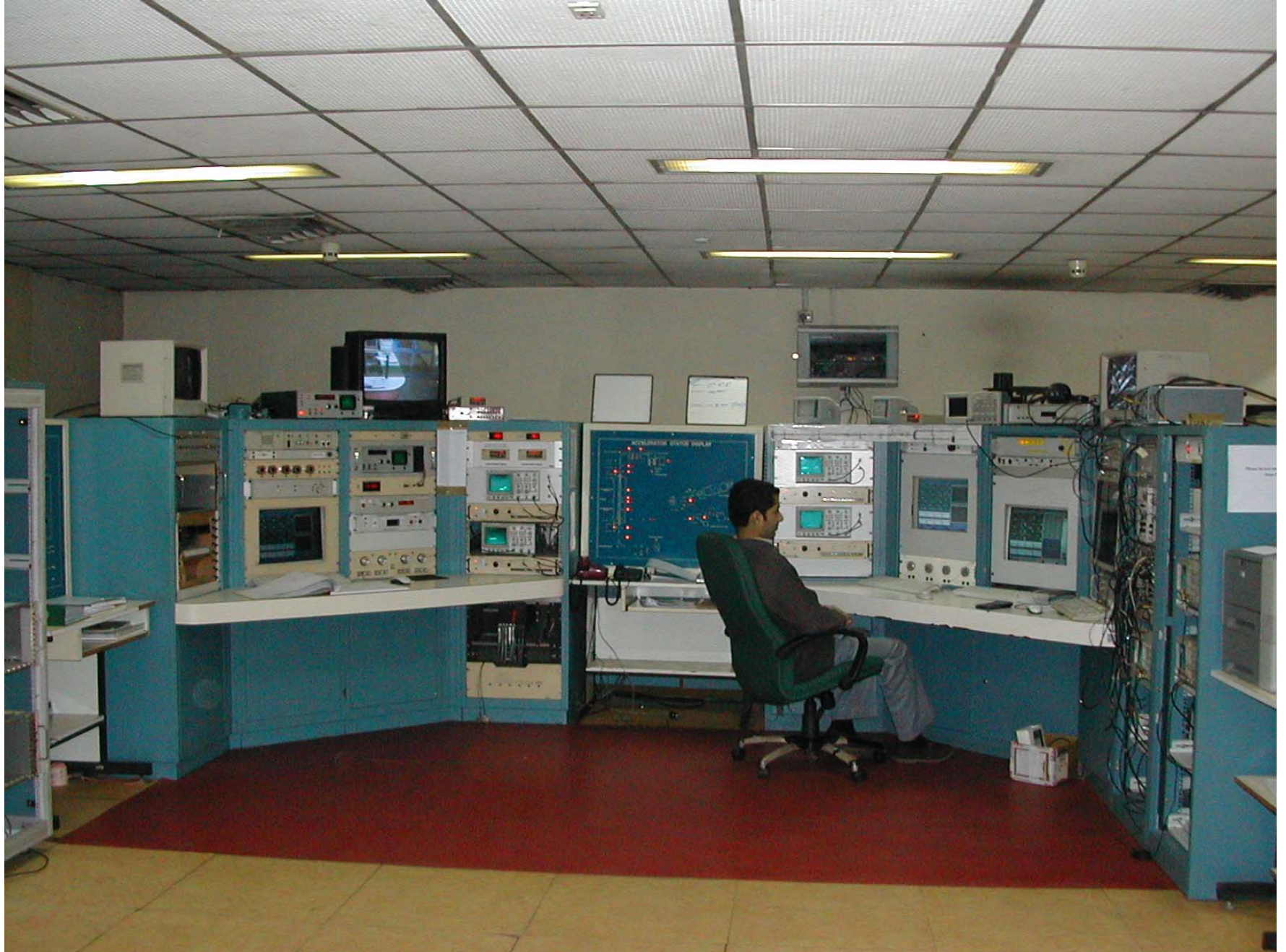
Control Room for 15UD Pelletron and Linac
